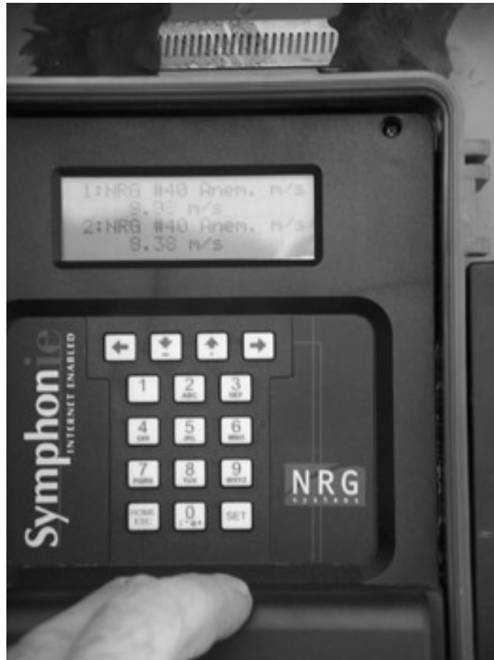
An NRG data logger is installed at the meteorological tower in Falmouth, MA. Data from the tower is collected through the logger and aggregated once a month by a community representative.
