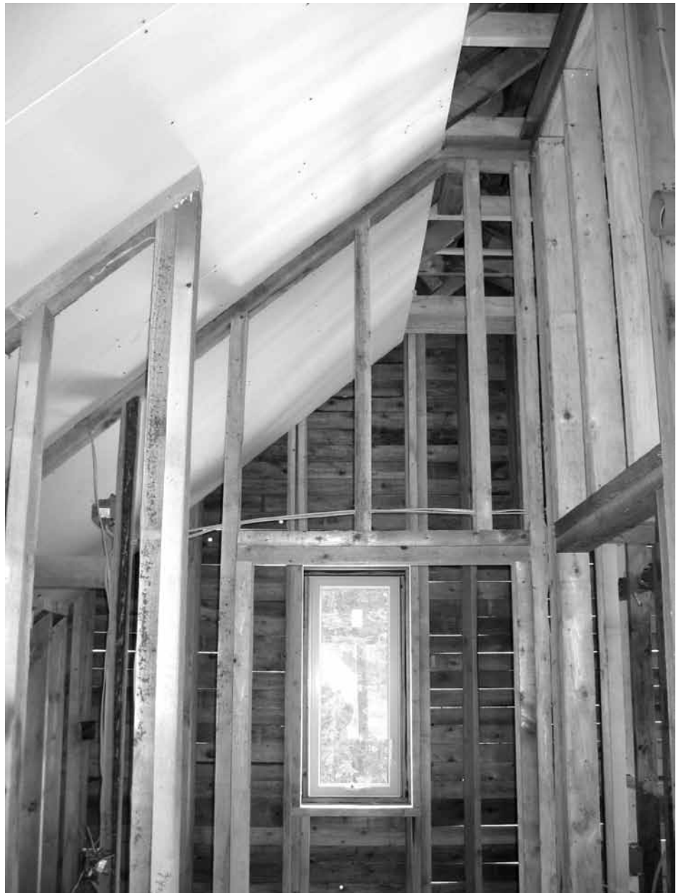
Cathedral ceiling drywall is put up before interior partitions are done, to reduce air leakage—drywall is the air barrier.
