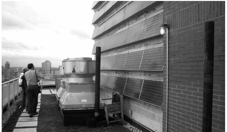
These solar panels would produce much more electricity if they were angled toward the sun and were not shaded by rooftop equipment. As installed, they represent a colossal waste of perfectly good solar panels.
