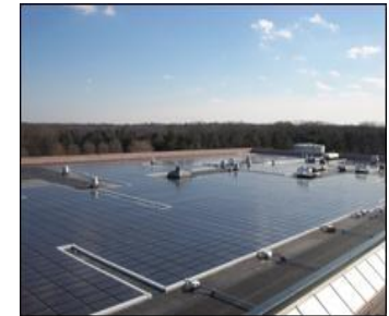
Solar PV Systems
