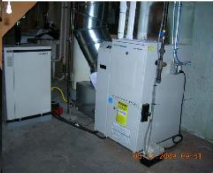
Freewatt Co-gen Unit
