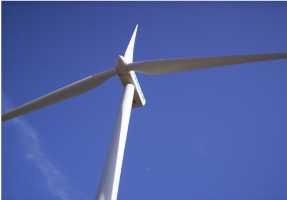
Hull Wind II, Hull, MA: Photo by S. Reyes
